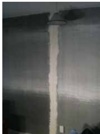
Once the plaster has dried, sand-back smooth to the wall surface. The whole walls surface now needs to be sealed using standard wallpaper 'Sizing'
